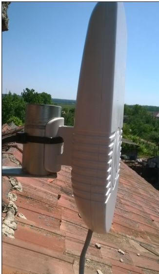
Station Module Provides Municipal Connectivity
